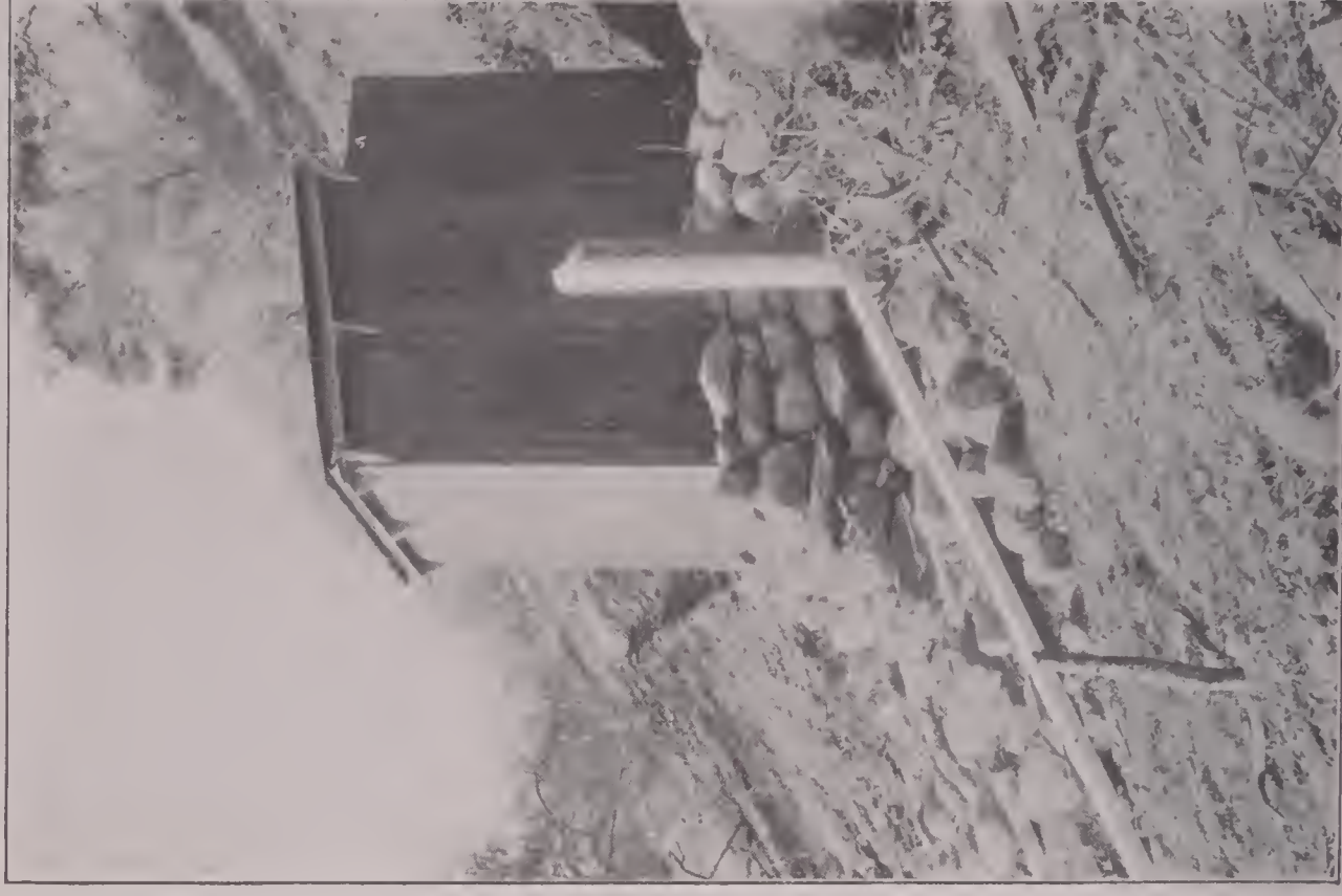
B. INCLINED AND VERTICAL STAFF GAGES BE-SIDE RECORDER INSTALLATION, SPOKANE RIVER AT POST FALLS, IDAHO.
